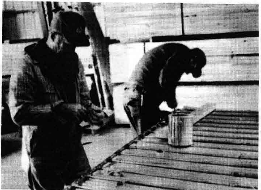
—Edgar Wuebben, left, and Linus Lange, both cooperators of the Energy Project, constructed one of the first solar water heaters at the Energy Project during the fall of 1977. Copper tubing is mounted to corrugated metal to provide the collector plate.
