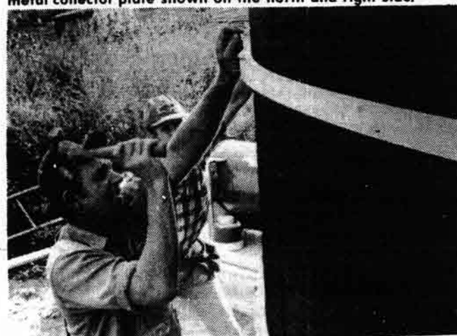
LaVern Truby, above, installs wood strips over the solar collector plate on his 6000 bu. bin, while Dennis Demmel of the Energy Project assists. The 1 x 2 wood strips were used to support a fiberglass cover. Similar wood strips were used under the corrugated metal plate. The strips were soaked with water for improved flexibility before bolting to bin.
