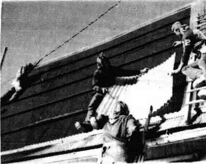
—Construction work underway on the Pinkelman solar farrowing barn. Fiberglass was placed over 2 X 2 purlins, which were mounted to the original sheet metal roof. The roof was painted black. Holes at either end of the roof are used to move air between the barn and the collector. Heat storage is located in the loft of the barn, which has a capacity for farrowing 22 sows at a time.
